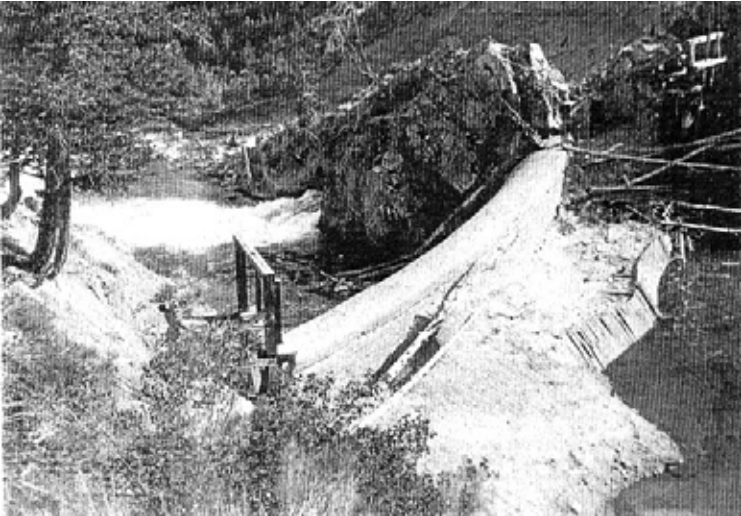
Sunbeam Dam before 1935. Upper right is the diversion tunnel gate; lower left, the power house tunnel gate.
