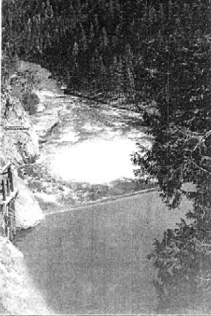
Rare view of Sunbeam Dam completely full with water flowing over the top. The white water in the center of the picture reveals the enormous pressure the high water creates in the tunnel.
